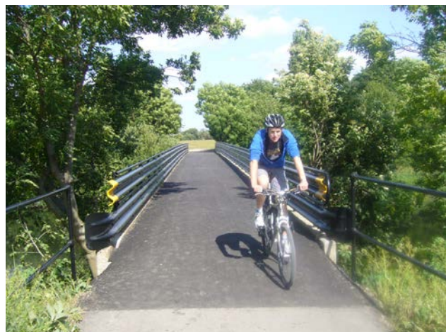
White House Lane bridge, Hackney – before and after. Conversion to a fit-for-purpose cycling link
